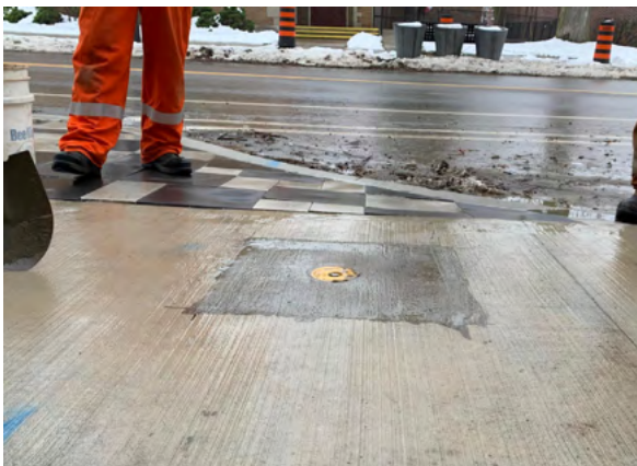
Gas valve box in sidewalk
